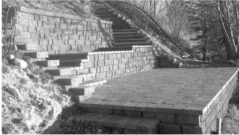
Guardrail missing or not installed (Patio)
