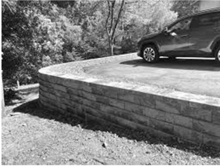
Guardrail missing or not installed (Parking Lot and Retaining Wall)
