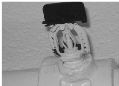
Sprinkler assembly has evidence of foreign material that is detrimental to performance
