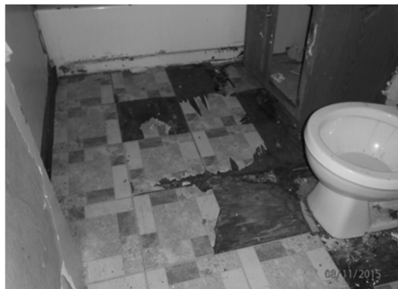
Rotted floor, almost fell through
