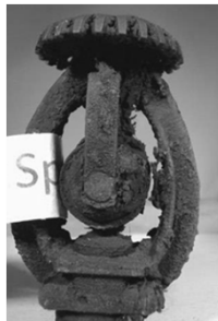
Sprinkler assembly has evidence of corrosion
